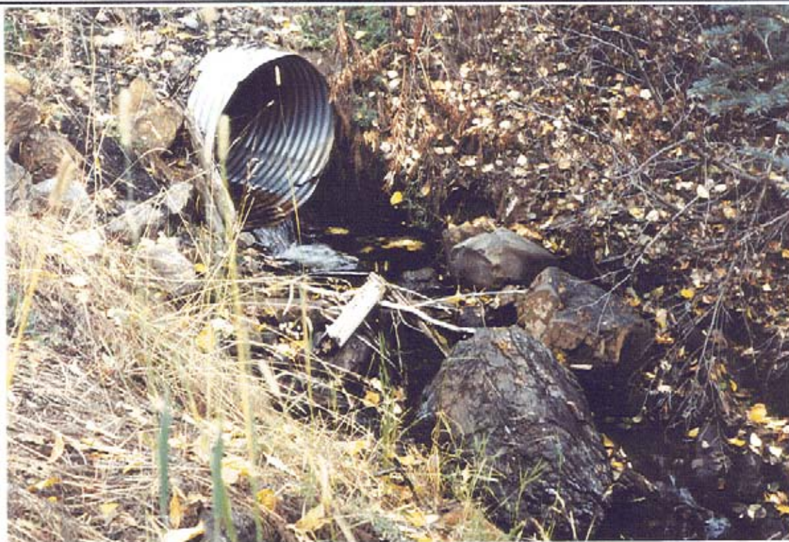
Trib 1, Reach 1, Site 2, 980m above mouth. Obstruction at road, especially to juveniles. October 10, 1996.
