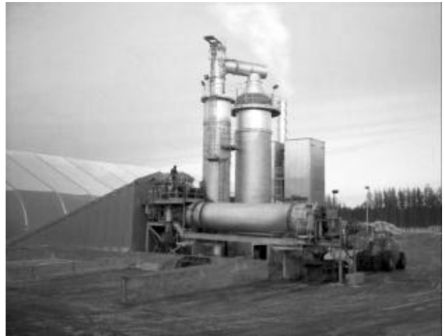
Photo courtesy of Bennett Environmental Inc.
